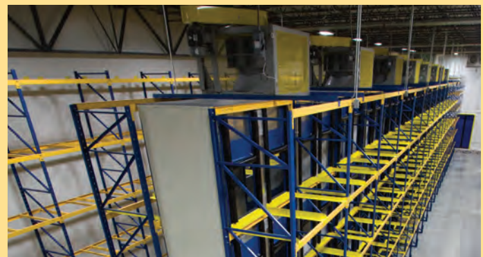
High-powered fans (shown at the top of this photo) are placed on top of each cell, which creates a vacuum chamber between two back-to-back racking configurations, forcing air to flow through the pallet spaces to create a more even freezing process.
